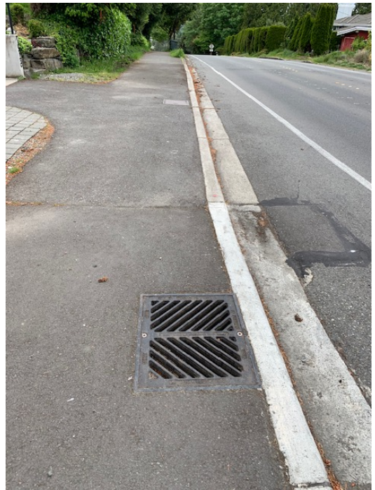
Catch Basin – Point F
