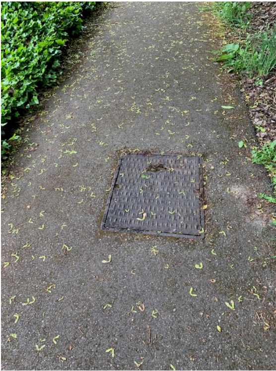
Catch Basin - Solid grate at H
