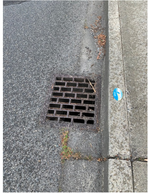
Catch Basin At Point S
