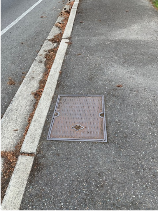
Catch Basin – Point G
